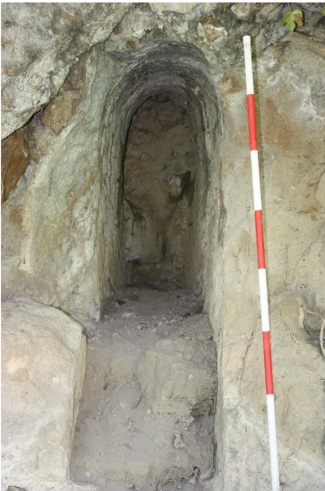
Fig. 10. Exit of late Republican aqueduct with remains of concrete vault viewed from the west, probably for outflow of water.
