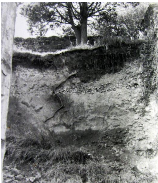
Fig. 3. Collapse at northwest corner. May 11, 1990.
