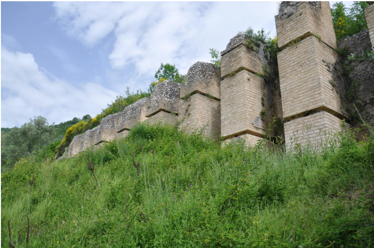
Fig. 2. Southern exterior of concrete terrace structure showing pilasters restored in the 1980s (Myles McCallum).
